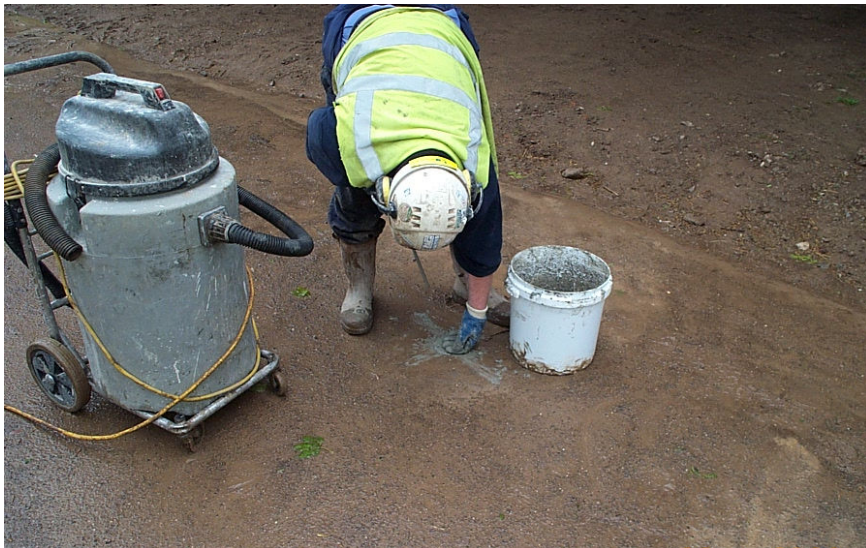
Figure 8. Vacuum used to clean out core holes prior to reinstating with concrete mix
